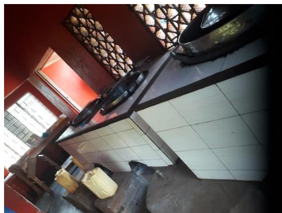
The new wood-burning stoves
