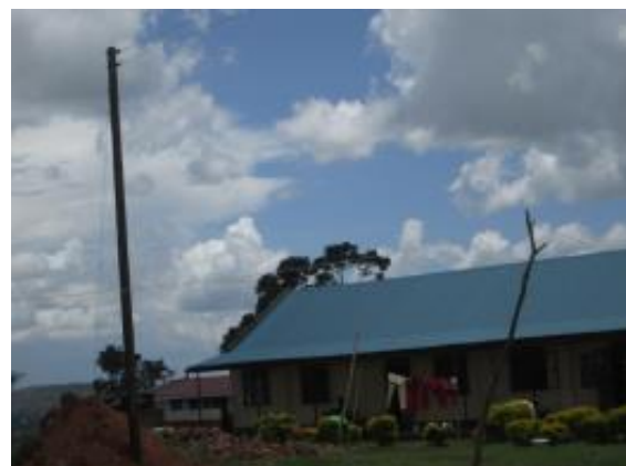
Electricity supply to main teaching block
